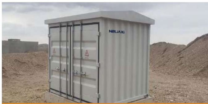
Australian outdoor energy storage cabinet system
