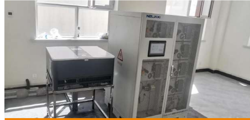
China Qinghai 30kW/100kWh energy storage system
