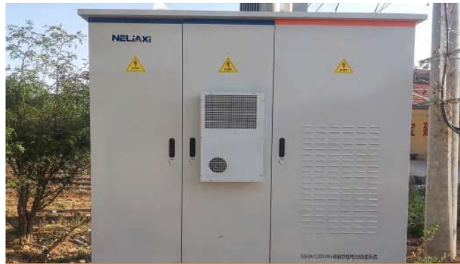
China Hebei 50kW/120kWh energy storage system
