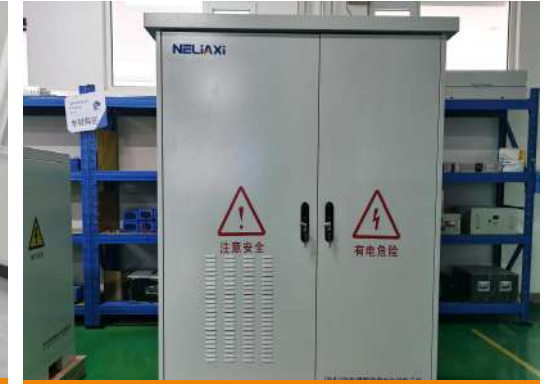
China Sichuan 50kW/100kWh energy storage system
