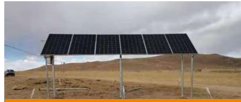
Pakistan Optical Storage System - 2 kW/12 kWh
