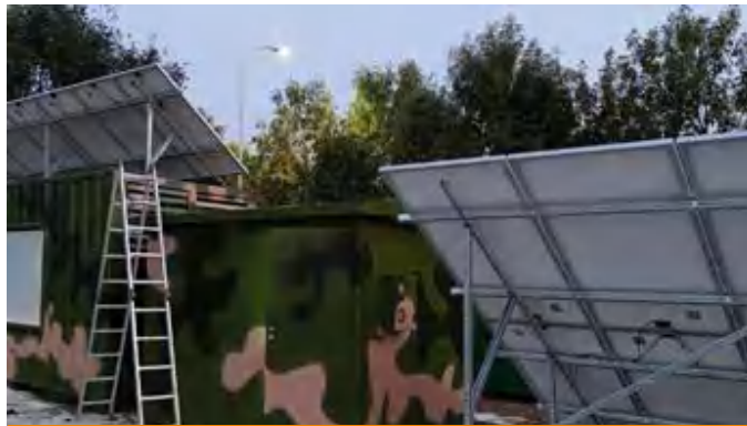
A military 150kW/200 kWh optical storage micro grid project
